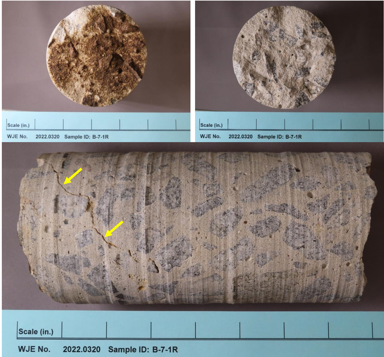
Figure A1. As-received appearance of exterior (upper left), interior (upper right), and side (lower) of Core B-7-1R. Separations within the exterior of the core are identified with arrows.
