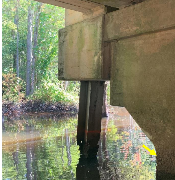
Figure 1. Bridge pier with corroded steel and deteriorated concrete near the waterline (arrow). Image provided by ESP.
