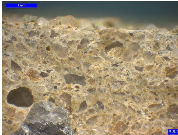
Figure 8. No distress in the concrete beneath the surface mortar on the surface of Core B-8-1.
