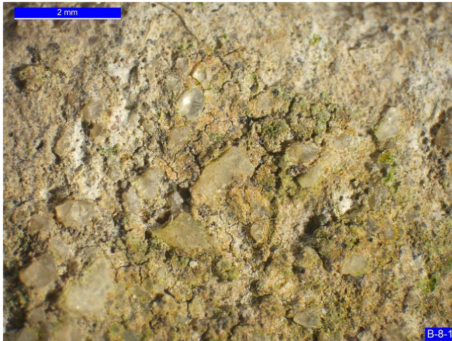
Figure A7. Green plant growth and microcracks on the surface of Core B-8-1.
